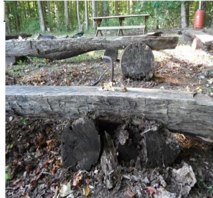
The rotting bases under the benches will be replaced.
